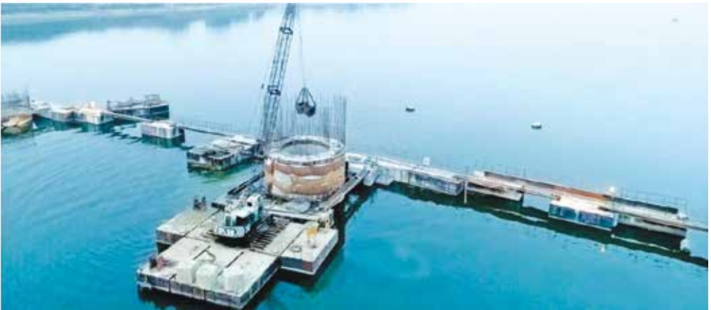
EDFC -Drone view of construction of bridge on river Yamuna at Prayagraj (Allahabad).
