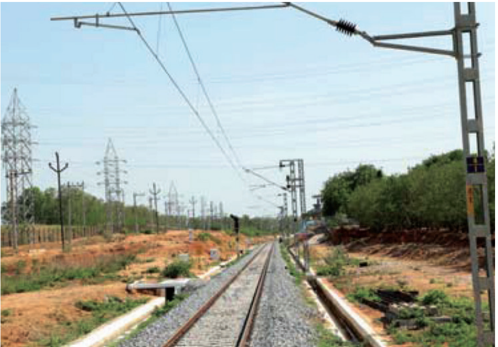
New Railway line with Electrification between Telapur-Ramachandrapuram facilitation suburban services in twin cities of Hyderabad, SCR
