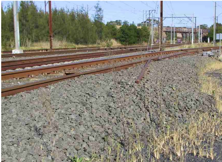
Figure 3 – Example of catchpoint with poor landing zone
